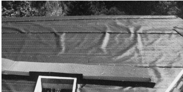
Conventional organic felts can absorb moisture, causing severe buckling and wrinkling.
